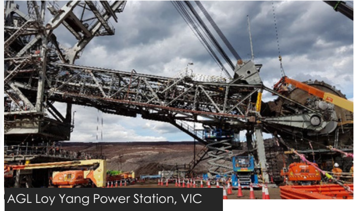
AGL Loy Yang Power Station, VIC Services: Engineering Survey of bucket-wheel dredger
